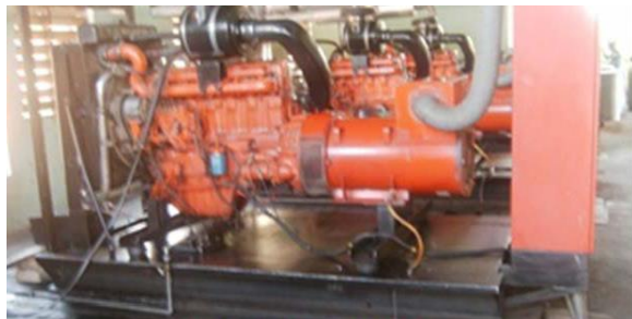
Figure 5: One of the 3 Diesel Generators in Likoma
